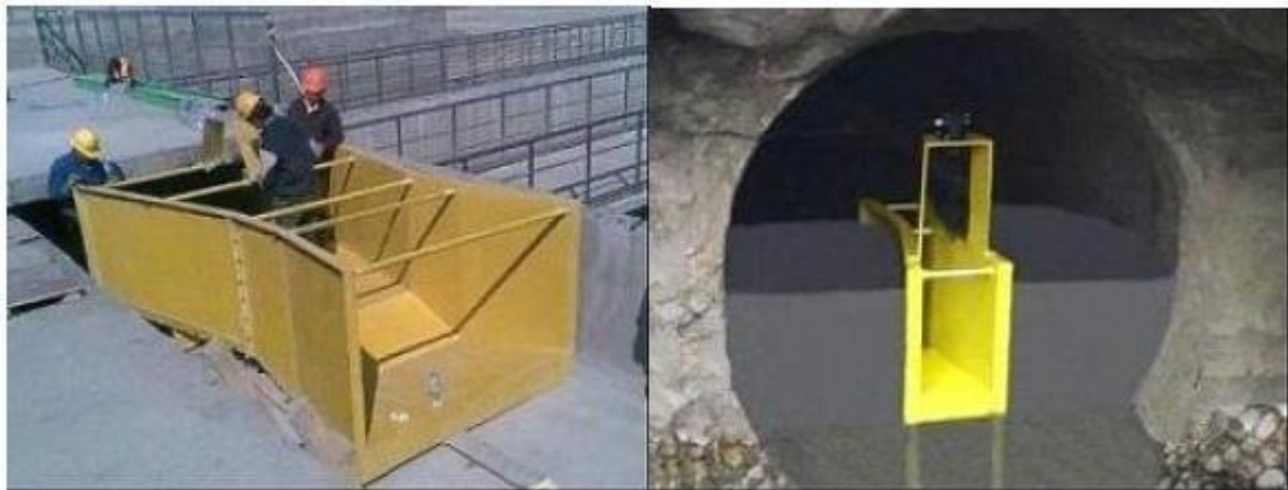
Parshall flume local installation pictures
